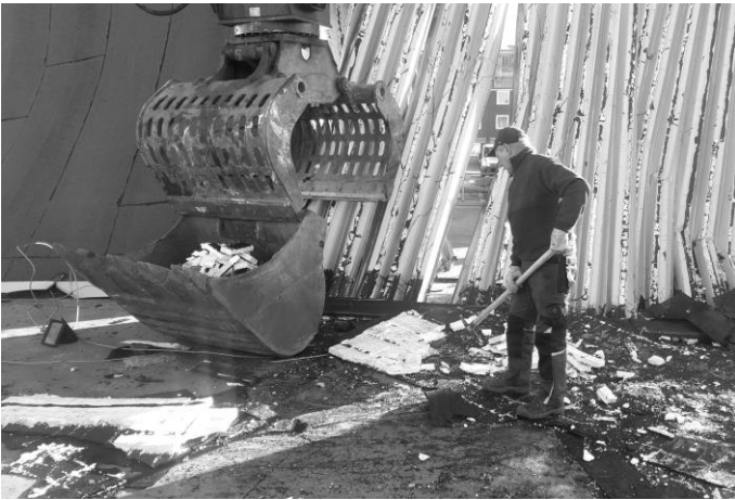
Figure 4. Hybrid element consisting of steel, foam and cardboard. All materials are glued together. With help of excavator-work, the steel can quite well be separated from the foam / cardboard. To remove the foam from cardboard, man-power is needed. Such difficult separation processes tend to increase demolition costs.
