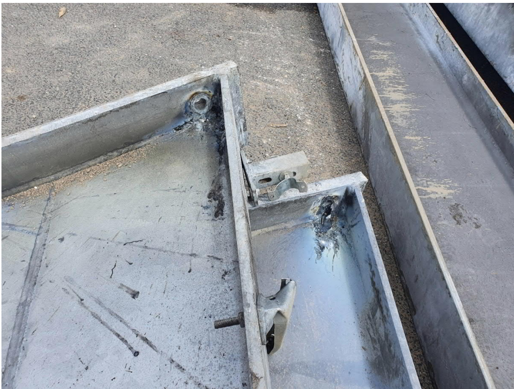
Figure 29: Detail: Small damage due to flame cutting.
