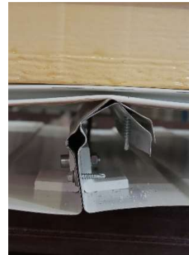
(b) Detailed failure mode
