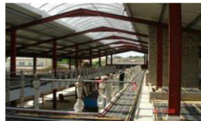
BCSA headquarters, Carwood Park, Doncaster, UK
