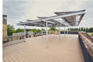
The Entopia Building PV canopy, Cambridge, UK
